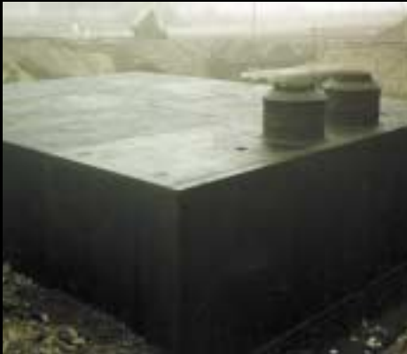
Water Storage Tank
