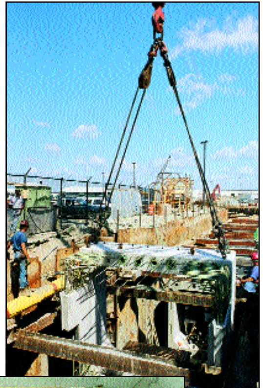
▶ The 40 ton pieces were lowered in-between the cross bracing and slid into place.
