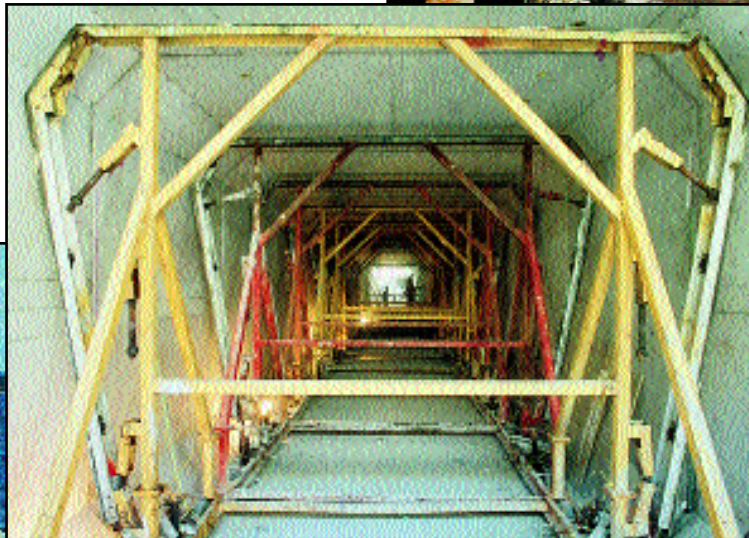
▶ Rotondo designed and built rubber covered rolling frames that formed the shear-keyed segment joints to facilitate field grouting.
