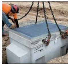
Microcell & Fiber Optic Vaults
