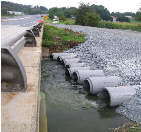
PA. State Rt. 272, Pequea Creek, Lancaster County PA, bridge bypass utilizing Oldcastle's 48" CL-4 RCP and the Kinsley's composite stone construction.
